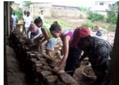
Students from the U.S. and Ghana work alongside local residents to rebuild wall of future community center.
