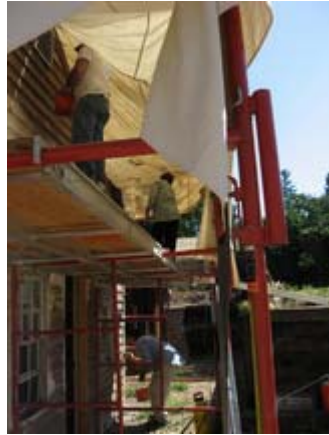
HCN participants learn how to prepare and apply historic finishes in Virginia City, where past, present and future all revolve around building preservation efforts.
