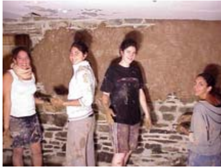
French students join their American counterparts in applying mud plaster by hand to the interior wall of the 1721 Hasbrouck House in New Paltz, NY.
